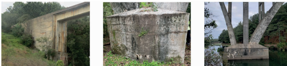
Figure 3 Substructure pathologies: concrete cracking, vegetation, concrete efflorescence
