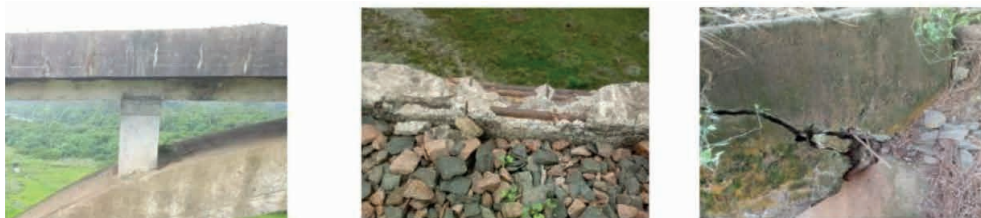
Figure 4 Superstructure pathologies: torsion cracks, steel corrosion, shear crack at Abutment B
