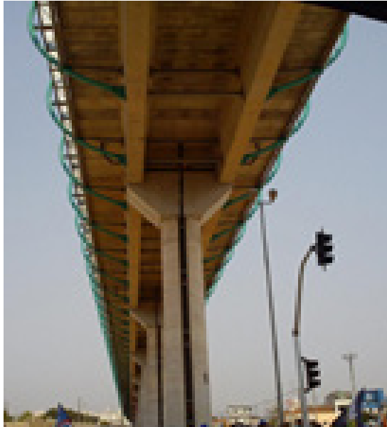
Figure AIII-5 - Example of a two lane elevated deck infrastructure for the LRT. Source: MECCA, 2013.
