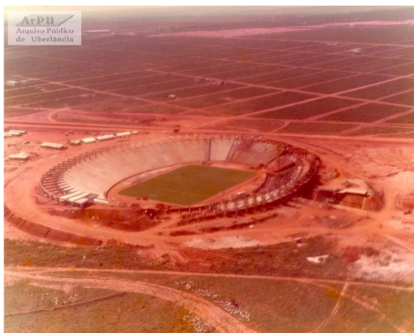
Figure 33 - Construction of the Sabiá Park Stadium, in the background of Santa Mônica neighborhood, 1970s, Uberlândia-MG.
