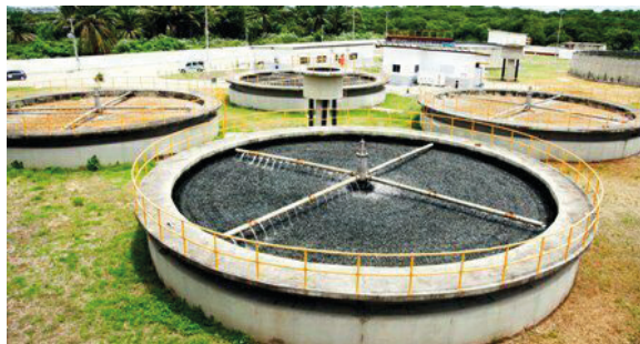
Figure 2: Dancing Days WWTP percolator filter (collection point for treated sewage).
