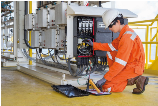
Figure 7.- Preventive maintenance of electrical installations https://www.jovalindustrial.com/blog/important-generator-maintenance-tips/
