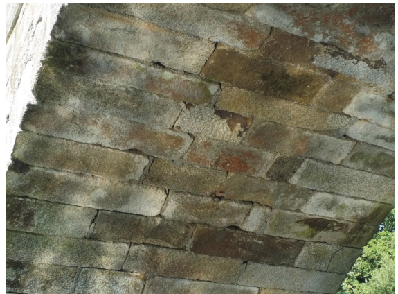
Figure 8 - General view of the downstream elevation of the Brandomil Bridge, in an image captured with the multi-rotor drone used in the inspection of this article (photo by the author).
