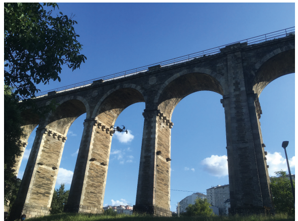
Figure 2 - Quadcopter drone approaching for an inspection over the Ponte da Chanca, a railway viaduct located in the city of Lugo, which celebrated its 150th anniversary on December 20, 2021 (photo by the author).
