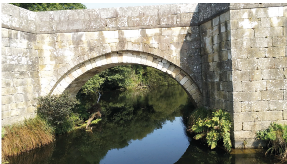
Figure 4 - General view of one of the major arches of the Bandomil Bridge, in image captured with the multi-rotor drone used in the inspection from the downstream side of the bridge (photo by the author).
