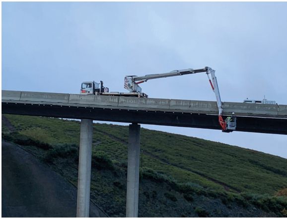
Figure 1 - Inspection of the deck of a viaduct that crosses the Rías Bajas Highway (A-52), at the height of the municipality of A Gudiña, in the province of Ourense (photo by the author).
