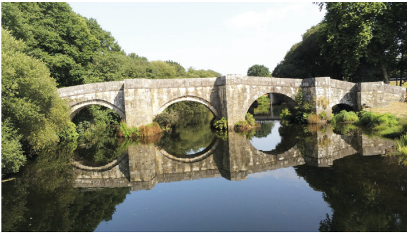
Figure 3 - General view of the downstream elevation of the Bandomil Bridge, in an image captured with the multi-rotor drone used in the inspection of this article (photo by the author).
