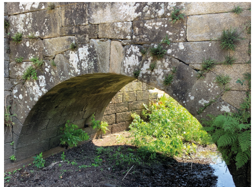
Figure 9 - General view of the smaller arch of the Brandomil Bridge, seen from the upstream side, in an image captured with the multi-rotor drone used in the inspection, where the abundant presence of vegetation rooted in the multiple elements can be observed (photo by the author).
