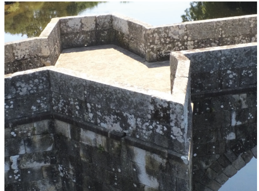
Figure 5 - General view of the upper part of one of the cutwaters of the Bandomil Bridge, in an image captured with the multi-rotor drone used in the inspection (photo by the author).
