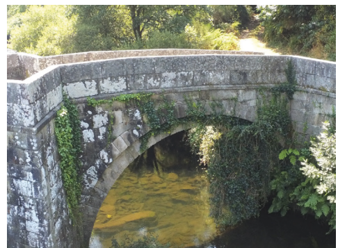
Figure 10 - view of one of the major arches of the Brandomil Bridge, seen from the upstream side, in an image captured with the multi-rotor drone used in the inspection, where the abundant presence of vegetation rooted in the multiple elements can be observed (photo by the author).
