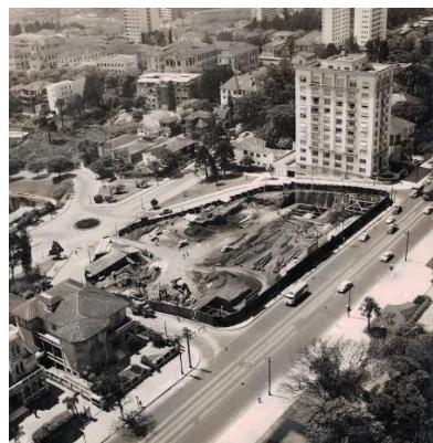
Figure 9: Lot 1578 on ``Avenida Paulista`` after the demolition of the first biennial pavilion
