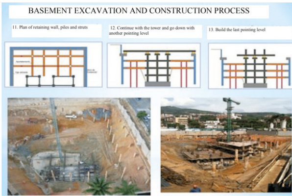
Figure 6: Excavation seen at the foundation level and the structure of the central core.
