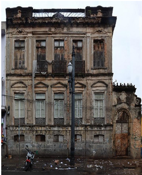
Figure 5: Photographic mosaic of the mansion's facade for the production of the Damage Map
