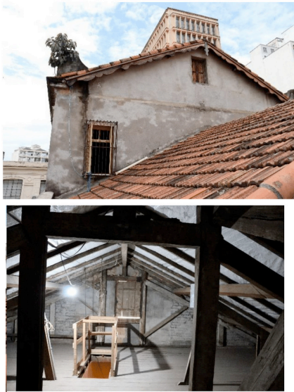
Figure 3: View of the roof in good condition and detail of the blanket placed below it
