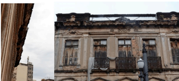
Figure 4: Facade elements where we notice plaster detachment
