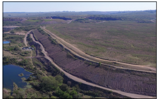
Figure 11: View of the tailings dam, covered and with revegetation on its surface.
