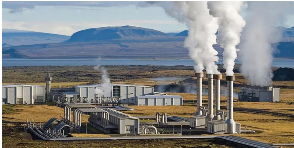
Figure 8: Geothermal Power Plant.
