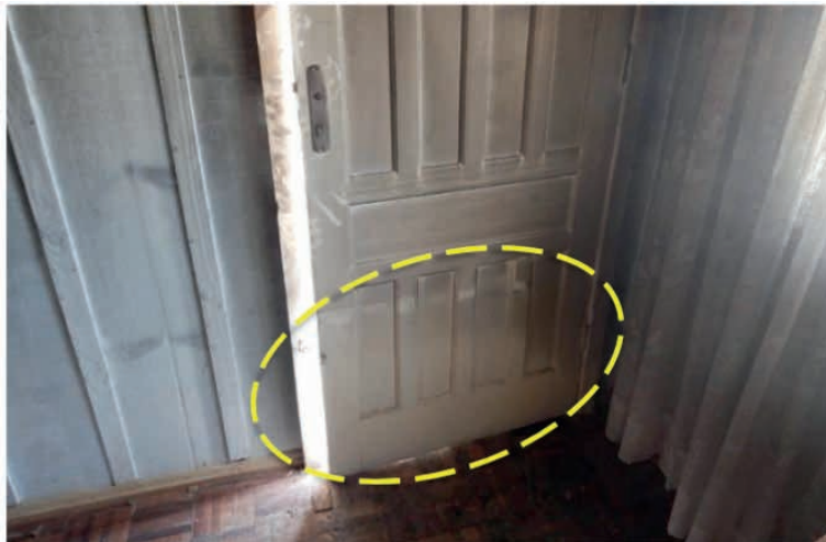
Figure 5. Shadow marks on the door
