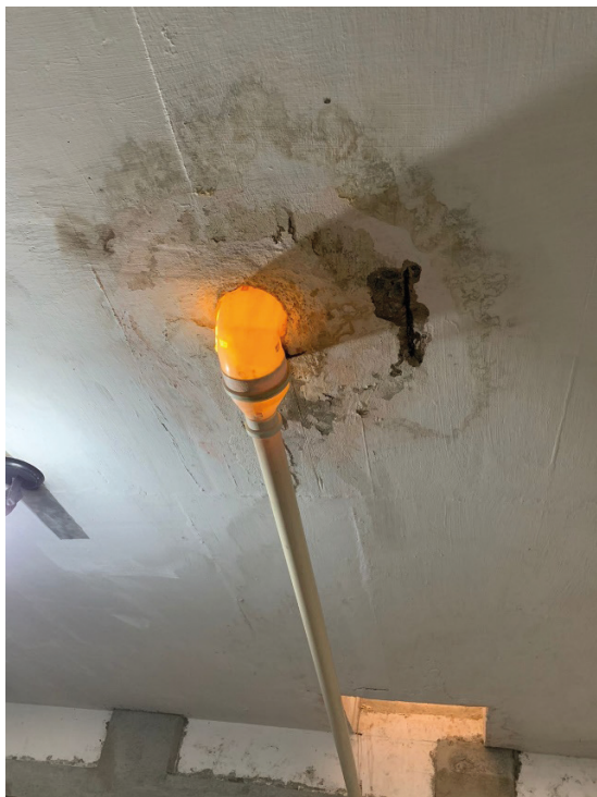
Figure 8 - Infiltration and exposure of reinforcement on the roof of the garage floor
