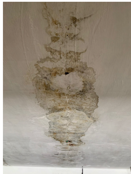
Figure 7 - Infiltrations in the ceiling of the garage floor with stalactite formations
