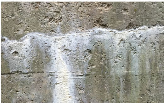
Figure 2 - Efflorescence on masonry wall [6]
