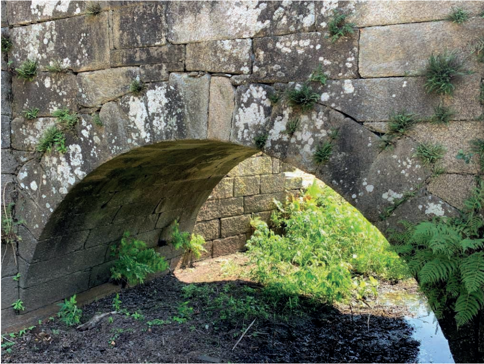
Figure 9: General view of the smaller arch of the Brandomil Bridge, seen from the upstream side, in an image captured with the multi-rotor drone used in the inspection, where the abundant presence of rooted vegetation can be observed in the multiple elements (photograph by the author).
