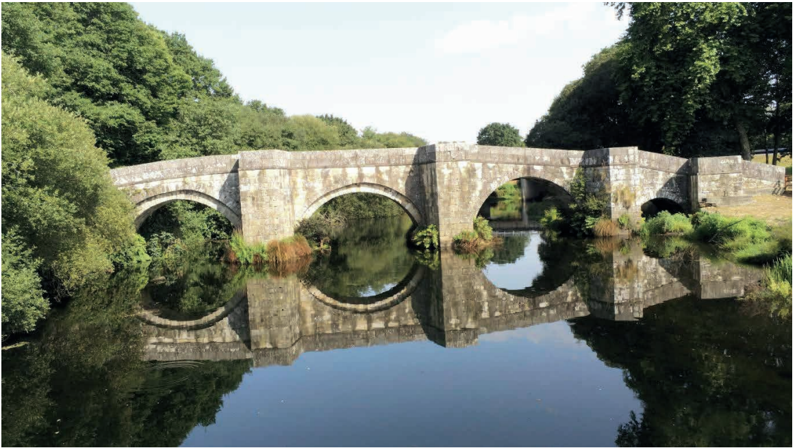
Figure 3: General view of the elevation downstream of the Brandomil Bridge, in an image captured with the multi-rotor drone used in the inspection of this article (photograph by the author).
