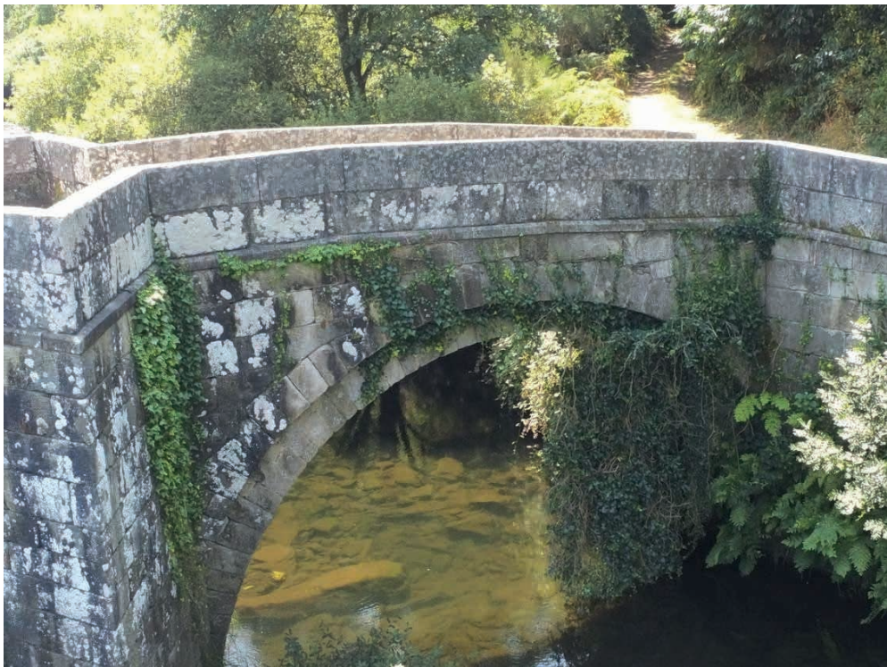
Figure 10: General view of one of the major arches of the Brandomil Bridge, seen from the upstream side, in an image captured with the multi-rotor drone used in the inspection, where the abundant presence of rooted vegetation can be observed in the multiple elements (photograph by author).
