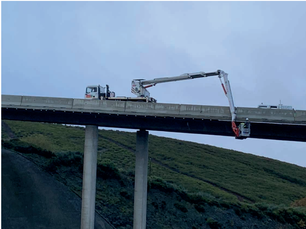
Figure 1: Inspection of the deck of a viaduct that crosses the Rías Bajas Highway (A – 52), near the municipality of A Gudiña, in the province of Ourense (photograph by the author).
