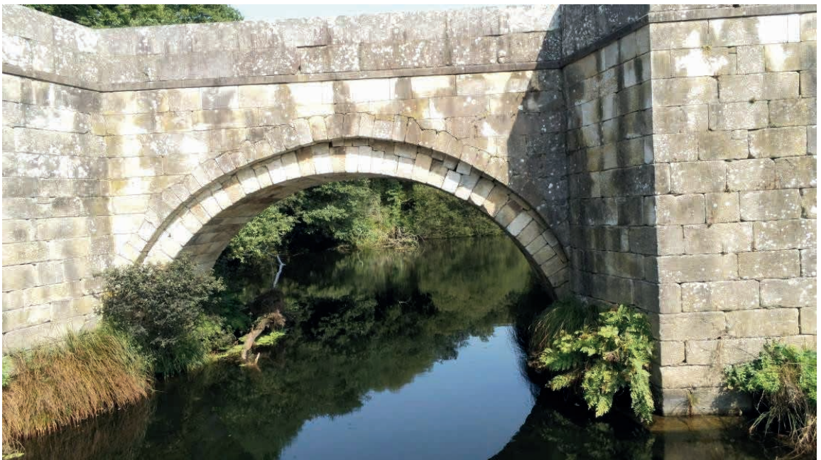
Figure 4: General view of one of the major arches of the Brandomil Bridge, in an image captured with the multi-rotor drone used in the inspection from the downstream side of the Bridge (photograph by the author).
