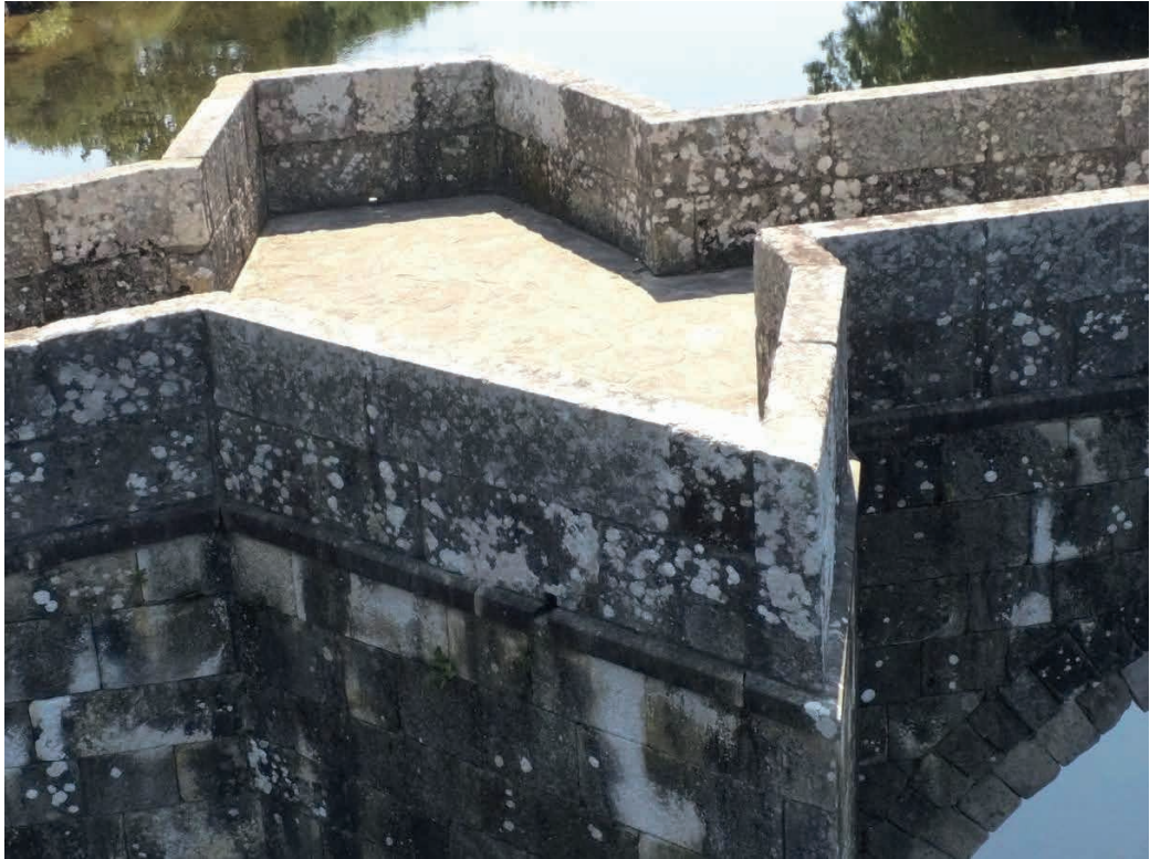
Figure 5: General view of the upper part of one of the cutwaters of the Brandomil Bridge, in an image captured with the multi-rotor drone used in the inspection (photograph by the author).
