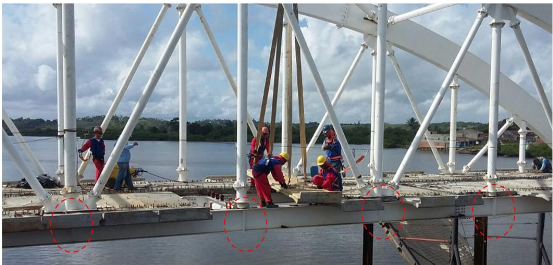
Figure 6 – Critical sections of the stringer beam regarding the occurrence of fatigue failures.
