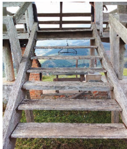
Figure 22 – State of conservation of the bandstand stairs. SOURCE: Author's collection (2022)
