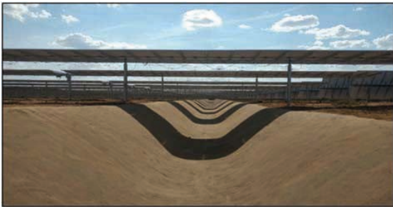
Figure 2.- Photovoltaic plant in Brazil. The largest plant in operation in South America.
