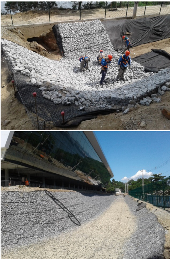
Figure 16 . Installation of the gabion mattress in the retention basin, November/December 2016. Source: Personal collection.
