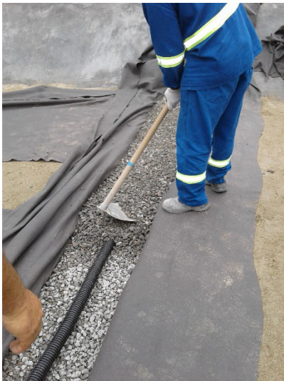
Figure 12 . Placement of crushed stone in the witness drain ditch in August 2016. Source: Personal collection.
