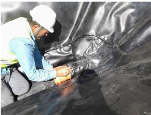
Figure 14 . Installation of a clamp to mount the waterproofing collar on the pipe in September 2016. Source: Personal collection.
