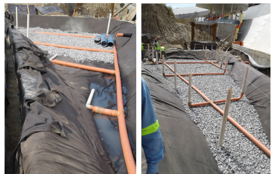
Figure 15 . Installation of hydraulic network and intercalated granular material, October 2016. Source: Personal collection.
