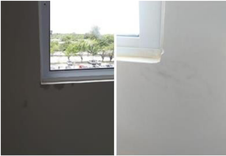
Figure 10. Infiltration at window frames (Construction Company Archive, 2020).
