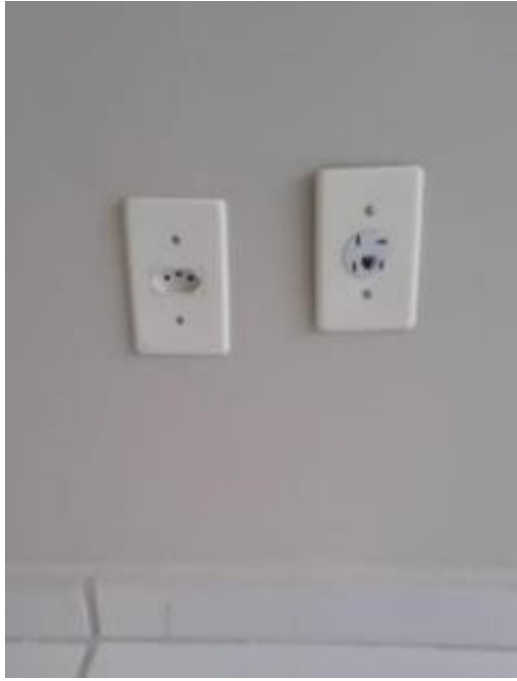
Figure 12. Misaligned electrical boxes (Construction Company Archive, 2020).
