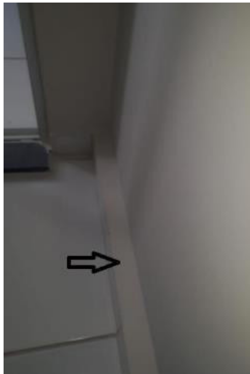
Figure 15. Out of square wall (Construction Company Archive, 2020).
