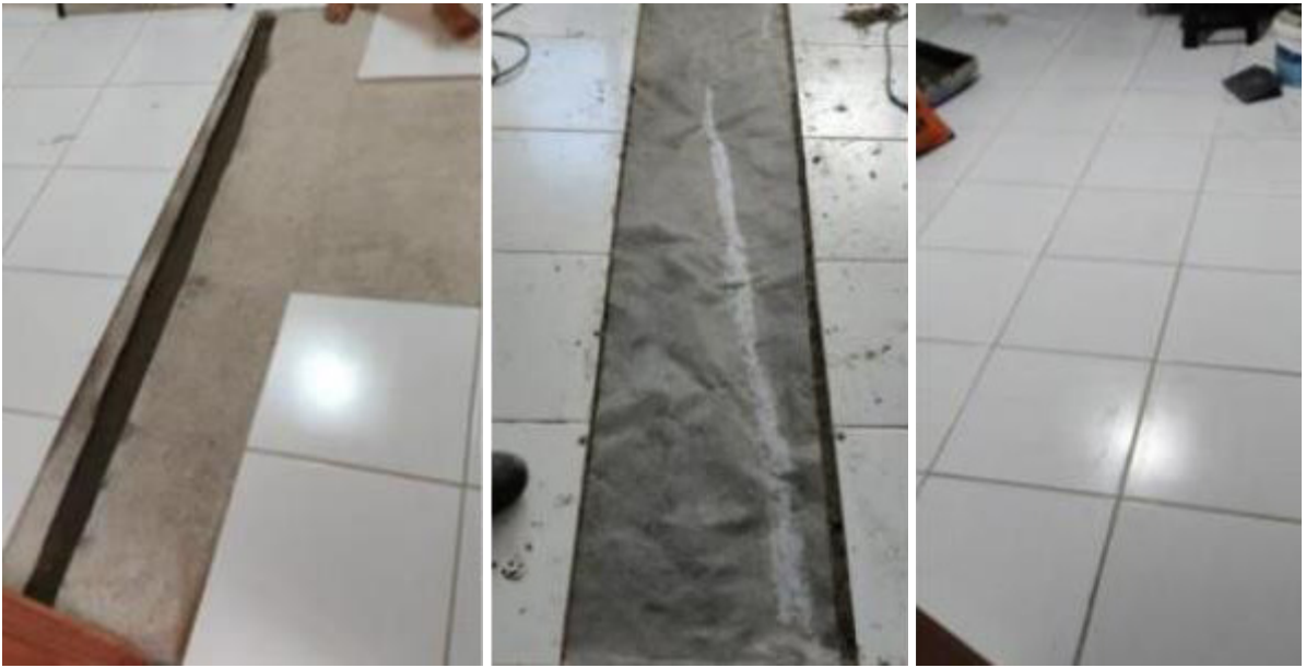
Figure 8. Correction of a crack in the floor due to a failure of the failure of the conduit cover (Construction Company Archive, 2020).
