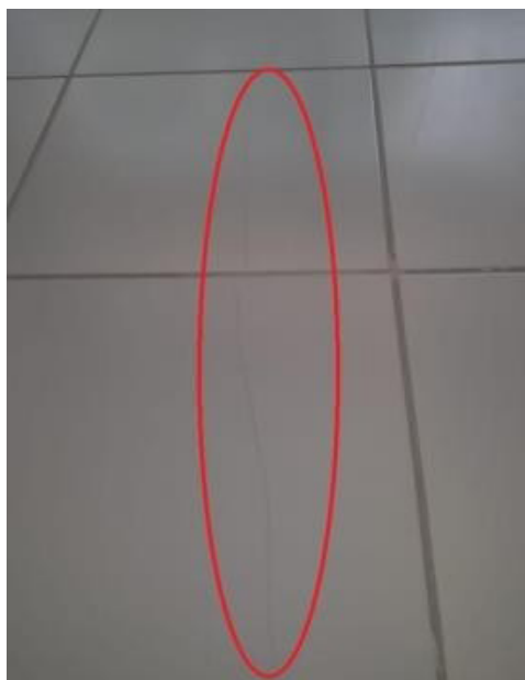
Figure 7. Crack in the floor due to failure in the covering of the conduit (Construction Company Archive, 2020).
