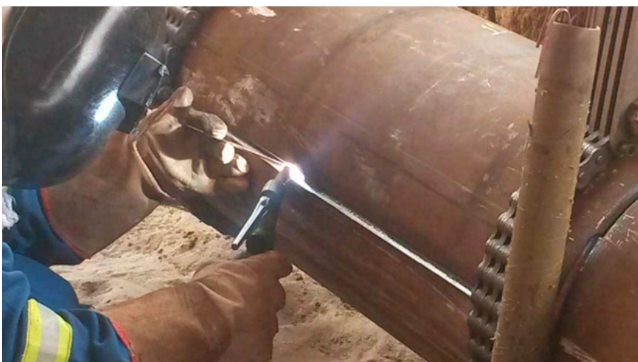
Figure 4 – Longitudinal welding of the root pass for the installation of the pressure-containing sleeves using the GTAW process – Gas-Shielded Tungsten Arc Welding [8].
