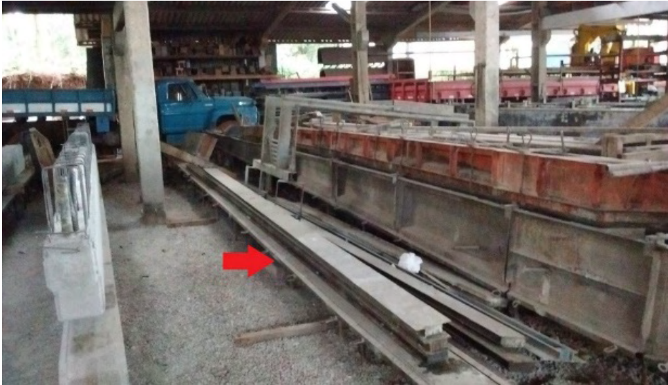
Figure 6 – Incorrect stacking of shape planks.
