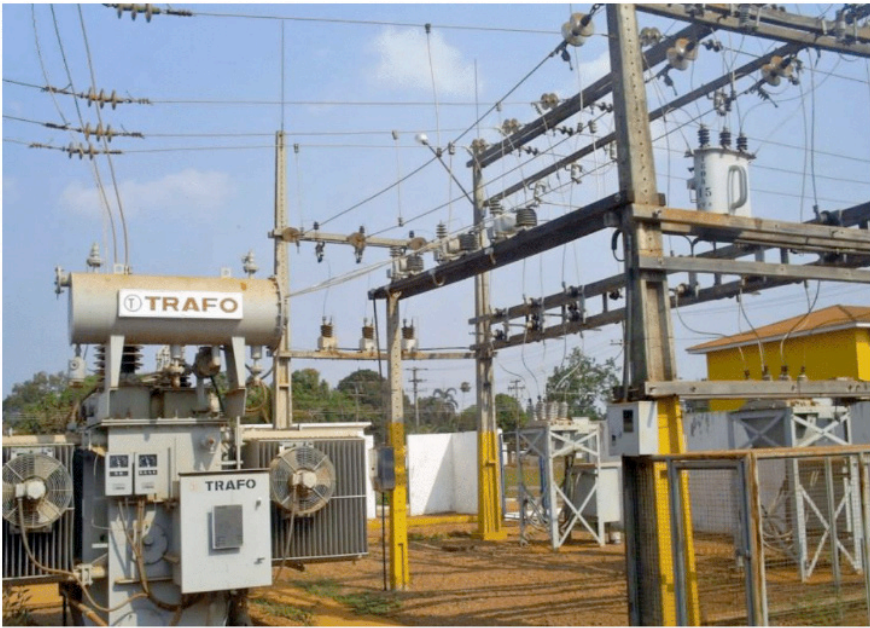
Figure 4. Distribution Substation of PRE Itapuã
