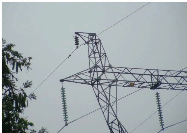
Figure 3. Detail of the lightning rod insulation at the top of the tower
