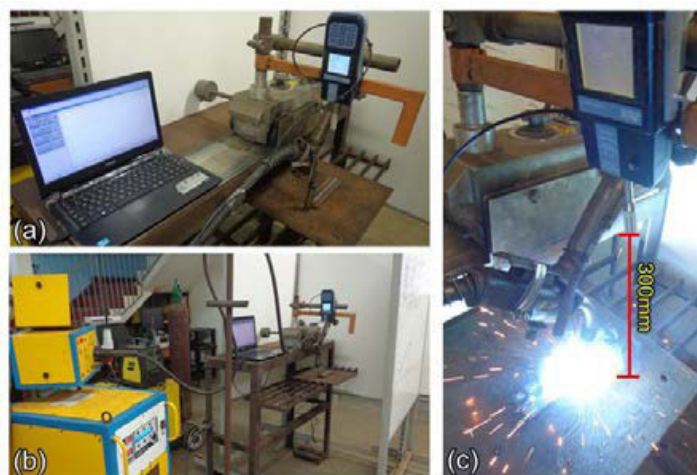
Figure 4. (a) Arrangement used to acquire gas concentration data. (b) Equipment positioning layout. The area was isolated with 3 welding screens. (c) Probe positioned 300mm above the welded part.
