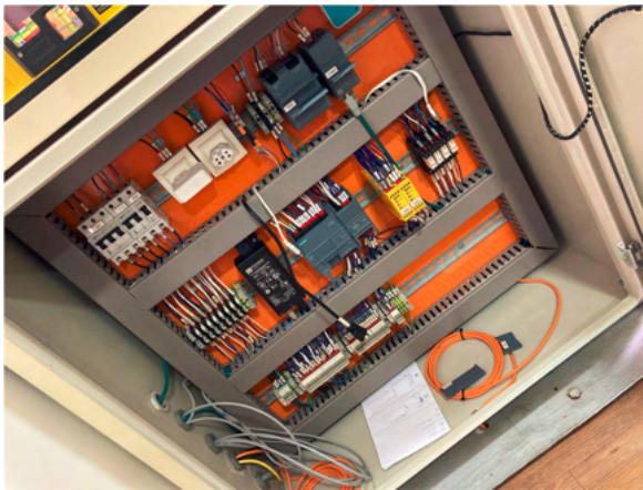
Figure 7. Electrical Panel for KUKA and ABB manipulator.
