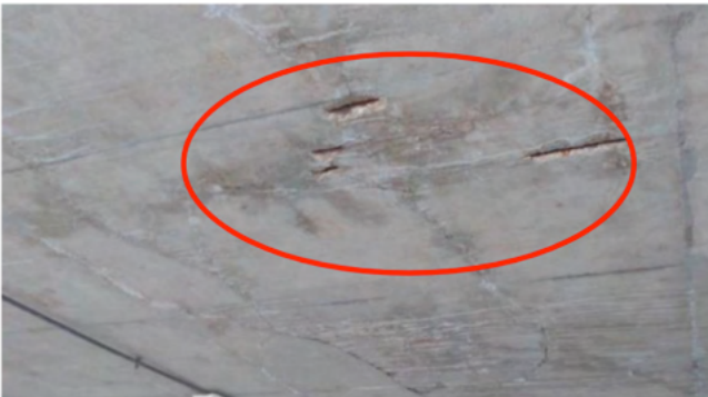
Figure 2. Concrete carbonation Source: Authors(2018).
