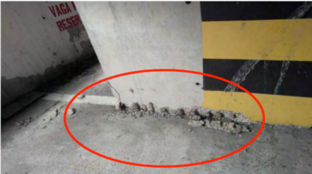
Figure 1. Corrosion of reinforcement at pillar base Source: Authors(2018).
